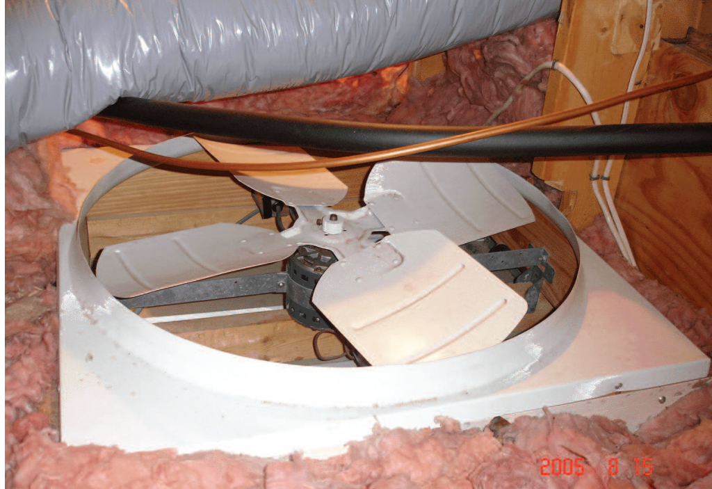
UNSAFE – potential for AC refrigerant lines and flexible insulated duct to contact the fan.
